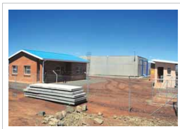
An office, reservoir and chlorination house – Maseru Water Supply Project
