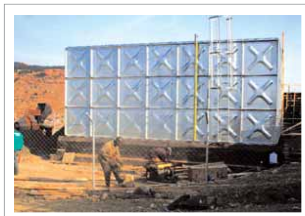
Construction of a reservoir at Ha Ratjomose – Maseru Peri-Urban Phase II Project
