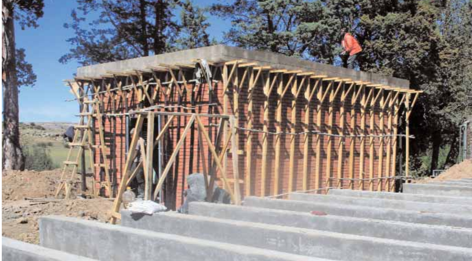
Construction of a pump house at TY, Three Towns Water Supply and Sanitation Project
