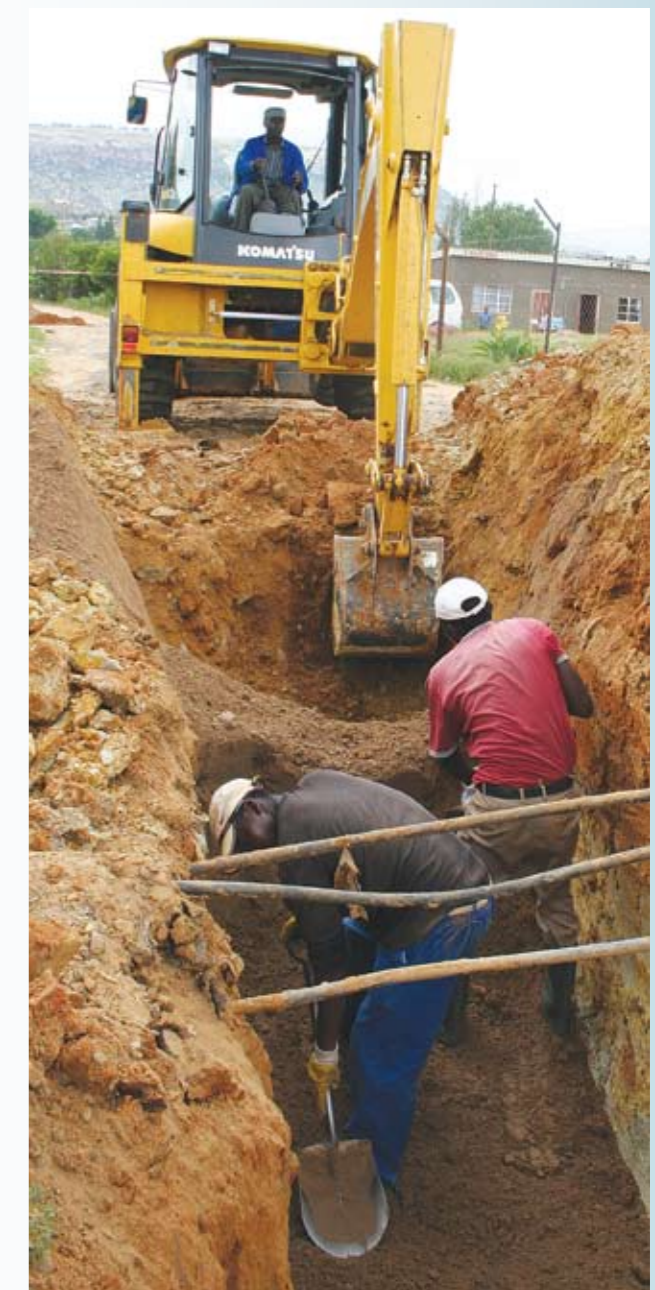
Trench digging for the laying of pipes at Naleli in Maseru City.
