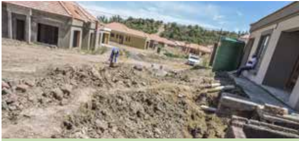
Khaho ea likoti tsa metsi a litšila ntle le Building Permit e baka ho khaoha h'a lipeipi, Maseru
