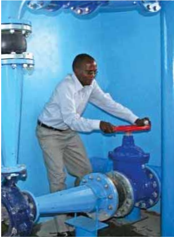
Molise Thabane Project Engineer for Three Towns Water Supply and Sanitation Project opening the water valve in the pump station
