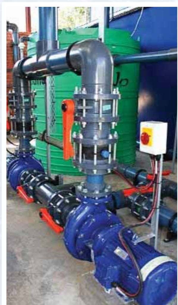
Quthing Package Treatment Plant
