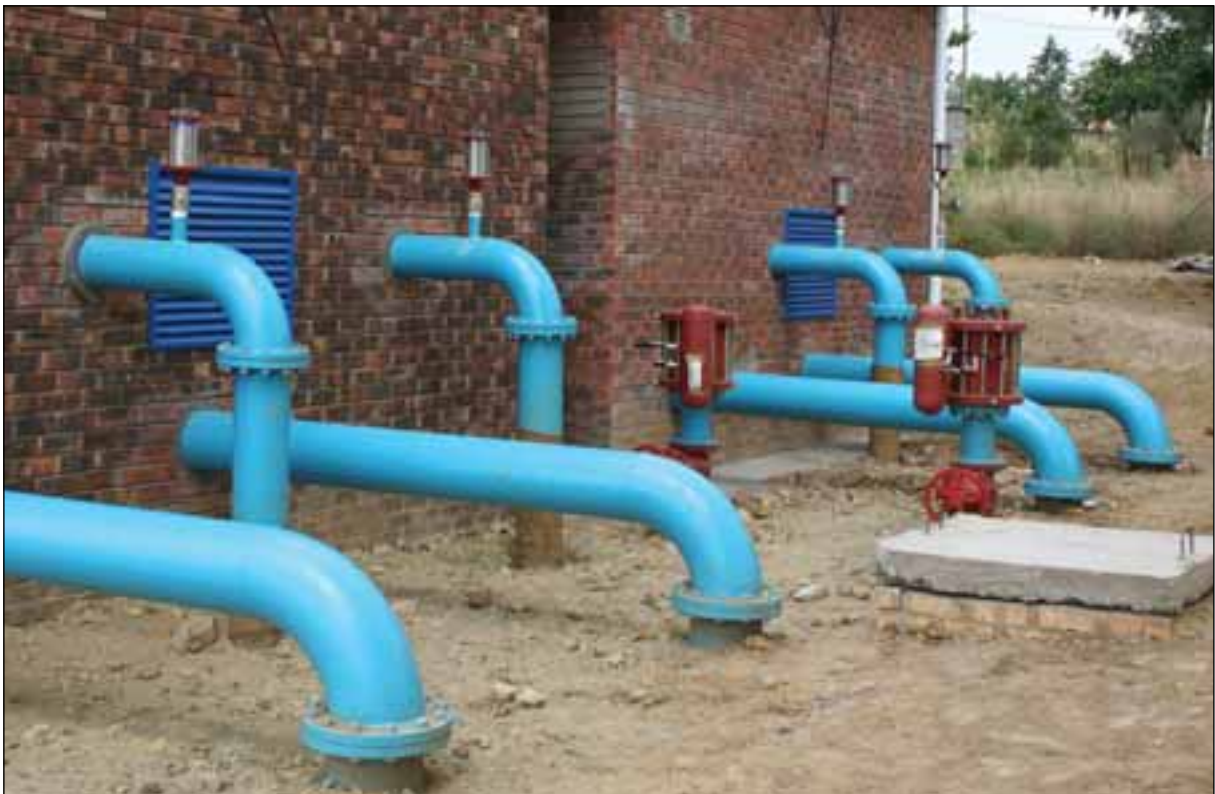
New pump station at Lithabaneng (Ha Motsoeneng)
