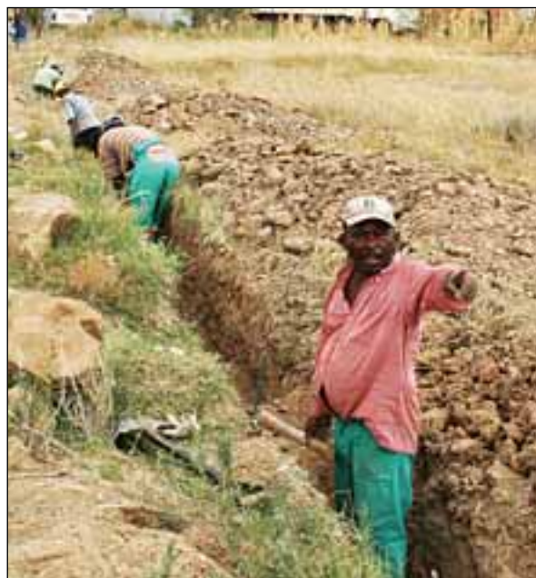
Digging of trenches at Ha Lesia for installation of communal pre-paid stand pipes.
