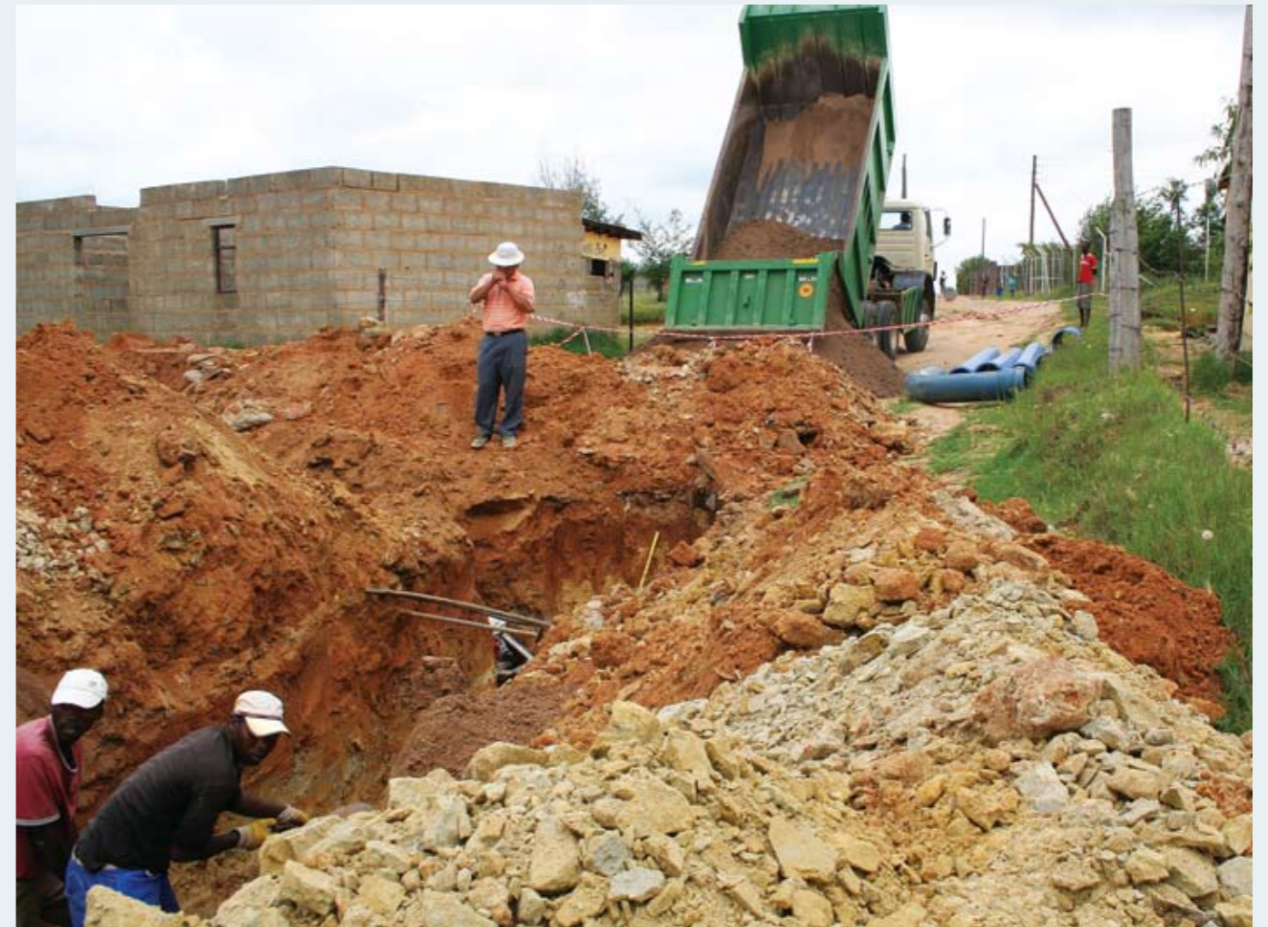
Maseru Peri-Urban Water Supply Project Phase II in the north west of Maseru City.
