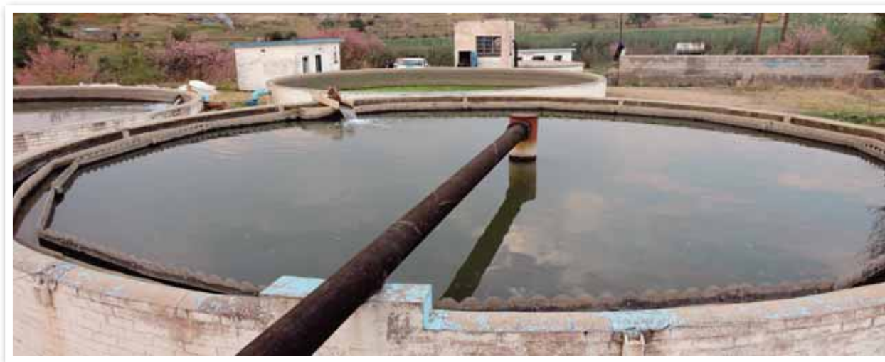
Sedimentation tank- Butha-Buthe water treatment plant
