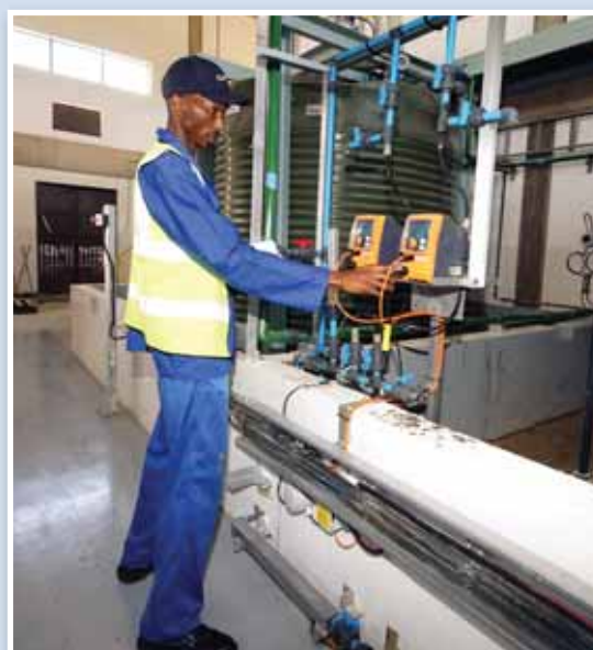
Plant operator operating chemical dosing pump
