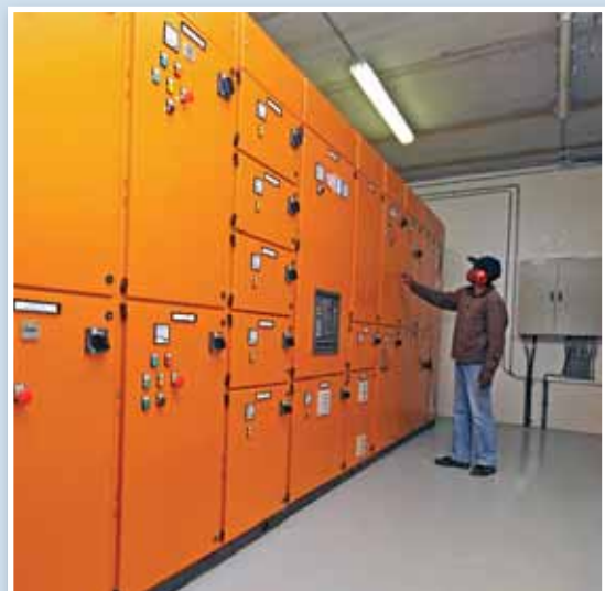
Operator operating control panel and VSD
