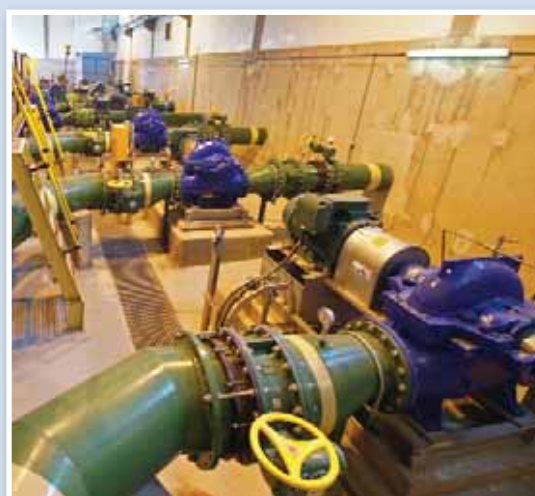
Lifter pumps used for backwashing filters
