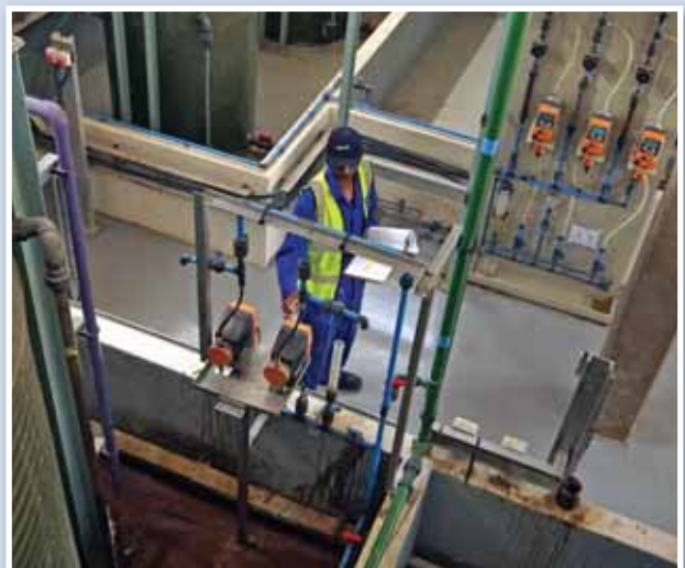
Metolong Chemical Room
